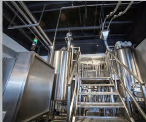
Brewing block for manual operation (5 hl, 10 hl and 17 hl)
